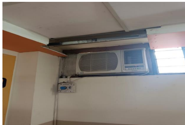
AC's provided inside the Campus
