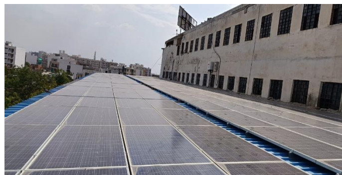
Solar Panel in the Campus
