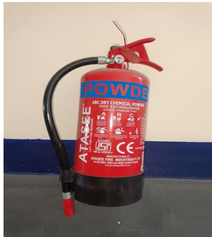
Fire extinguishers provided
