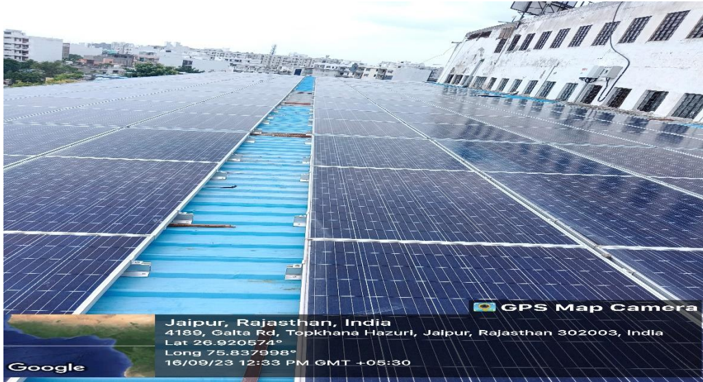
Picture 2 - Solar Panels Installed in the College Campus
