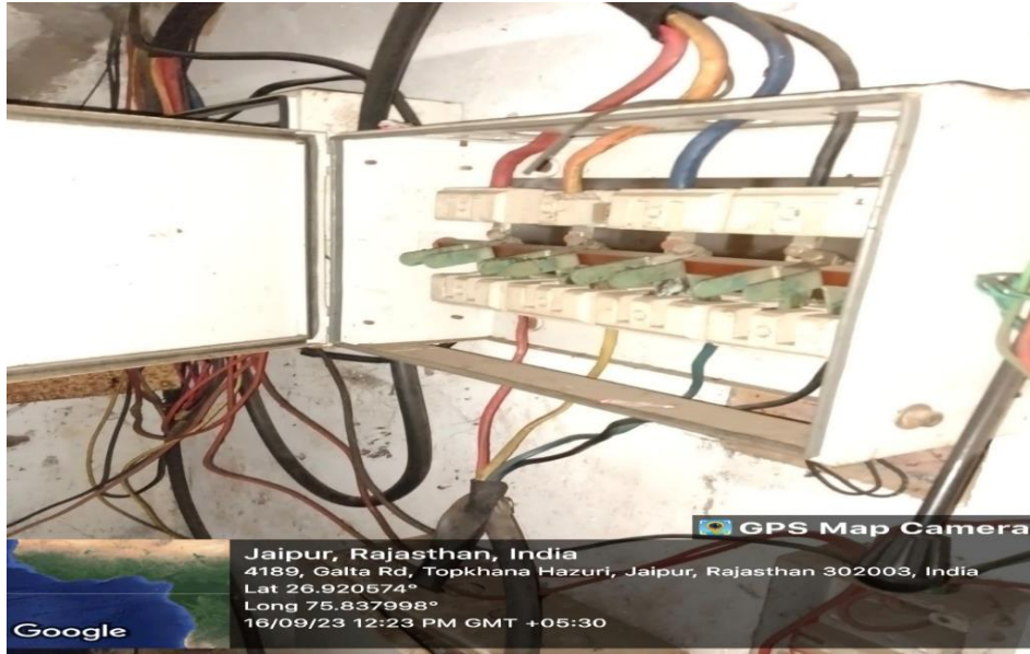
Picture 1 - Main Switch Control
