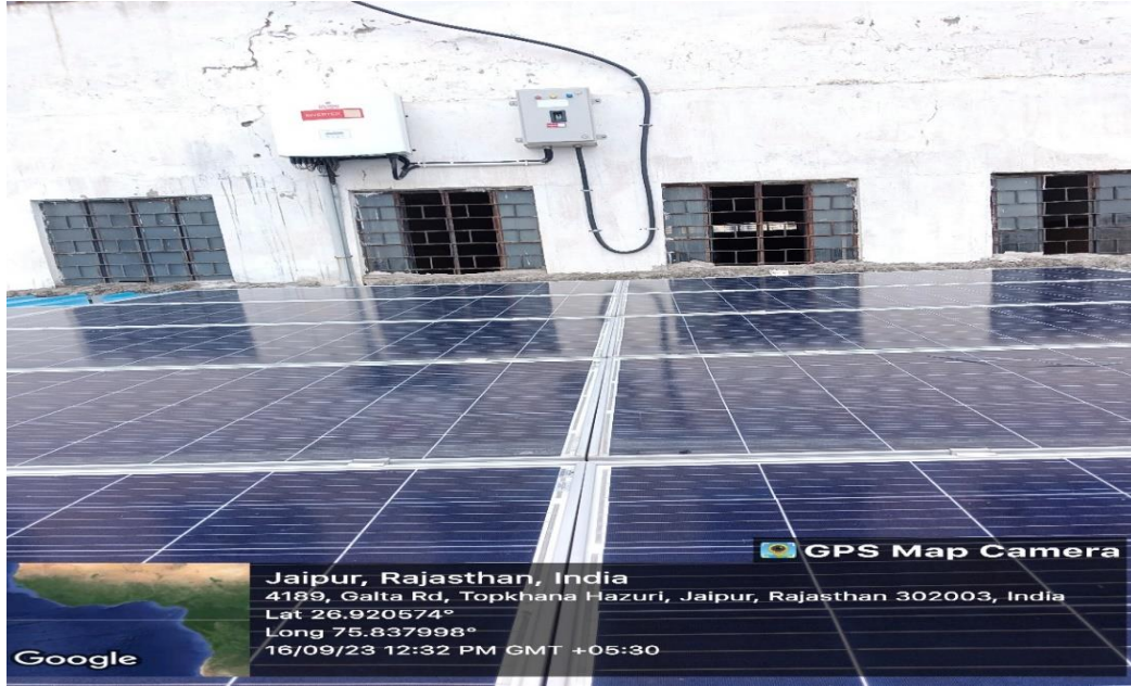
Picture 1 – Solar Panels Installed in the College Campus
