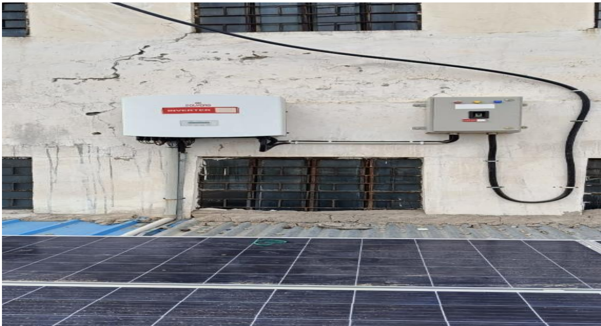
Solar Energy System in Campus
